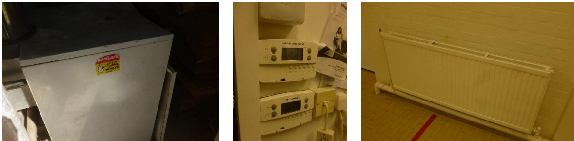
Figure 1 HVAC equipment (left to right) – ageing non-condensing boiler; heating system programmers are not fit for purpose; radiators in some cases are damaged
