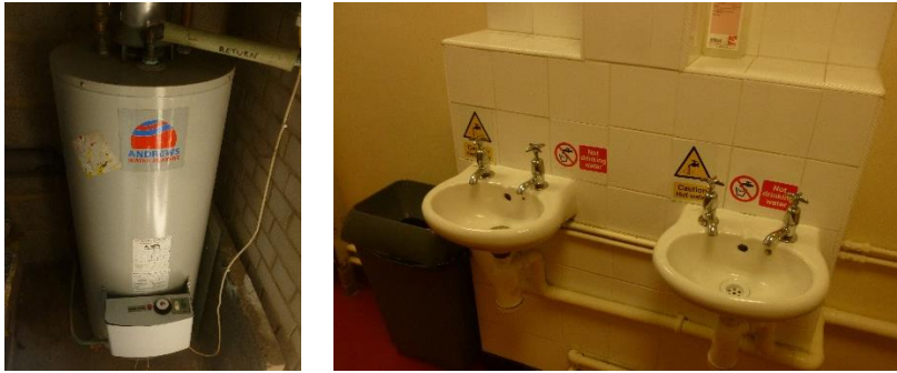
Figure 2 HWS equipment (left to right) – hot water heater struggles to meet demand; taps are not fitted with water saving devices
