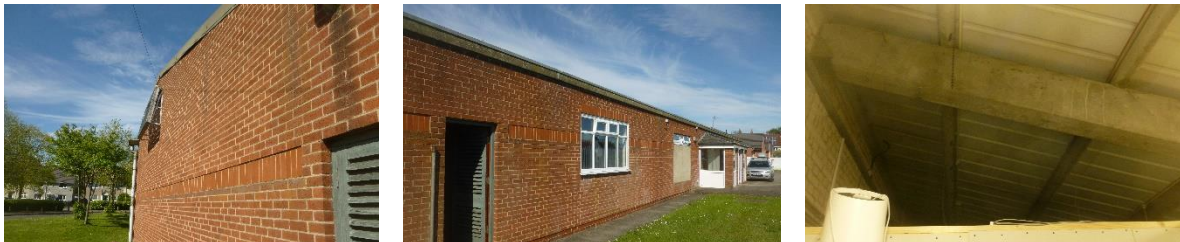
Figure 3 Building fabric (left to right) – cavity brick slips applied to original walls; cavity wall construction on frontage; underside of metal roof, no insulation as-built or above suspended ceiling
