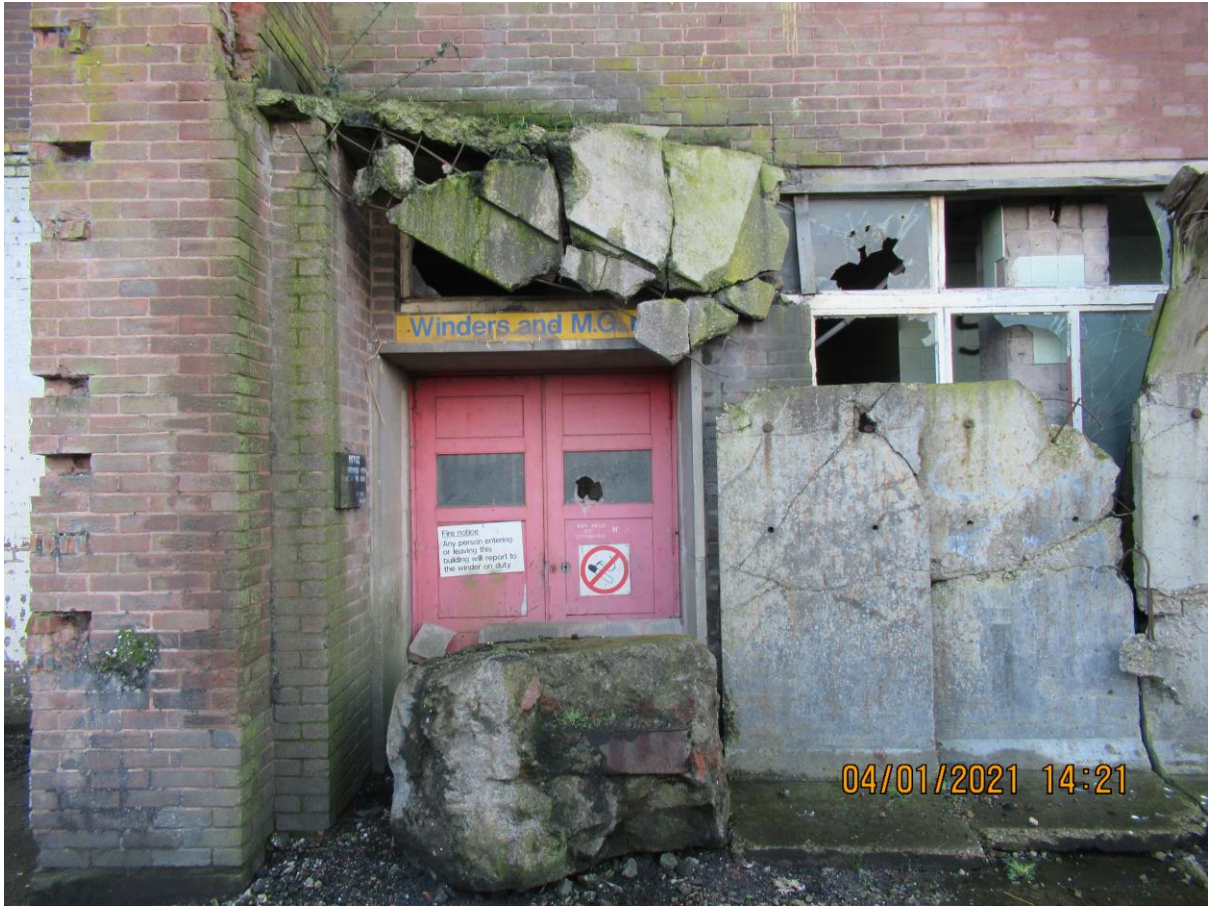
Picture above shows one the two pairs of red doors fitted either side of the main roller shutter door to the east side of the power house.
