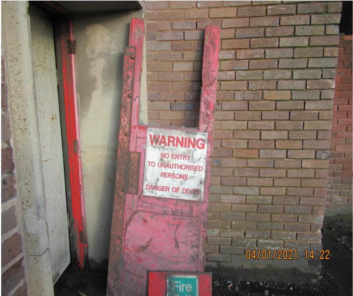
Picture above shows the damaged red door to the north end of the power house.
